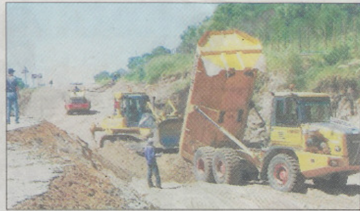
URGENT WORK: WBHO are working flat out to repair the R330 - from 5am till 10pm daily - with four dumper trucks, an excavator, loader, bulldozer and TLB. Picture: Yvonne Craig
